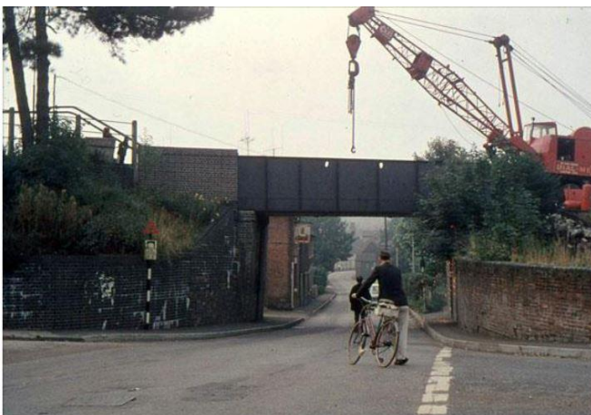
The bridges across Station Road and Waddling Lane were demolished in August 1967.
